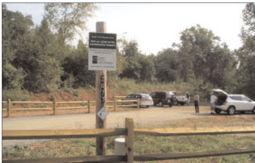
Work progresses nicely at the South Fork River Rail Trail, the Conservancy's first public access trail. The trail will open officially in spring 2005.
